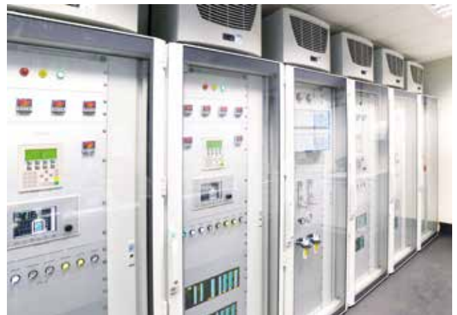
Control cabinet cooling
