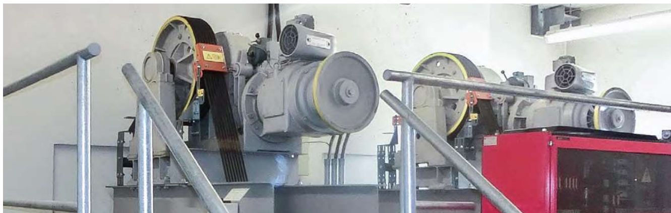
Old - Drive technology with gearbox and steel cables
